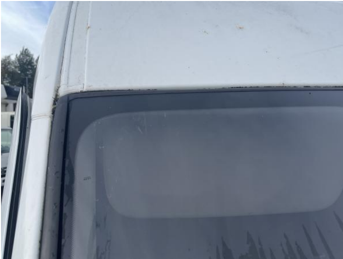
3: Roof Rusted Over 5mm
