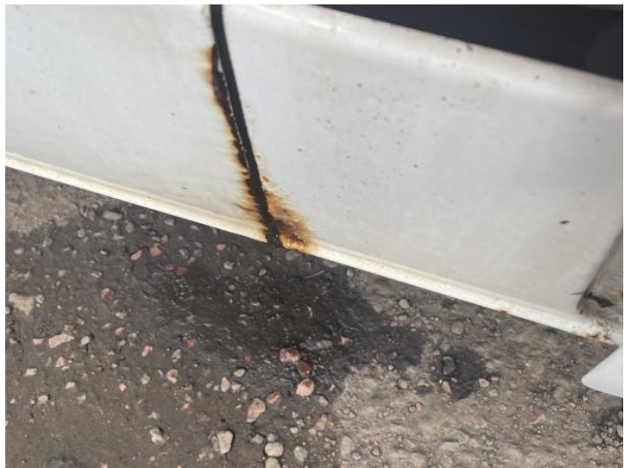
6: B Post os Rusted Over 5mm
